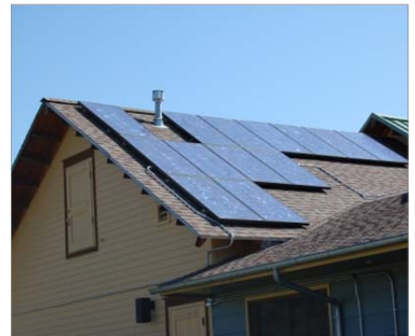
The Town has taken many steps to promote the efficient use of resources and to incorporate sustainable practices in its facilities and day-to-day operations, such as installing solar panels on Town Hall and other municipal facilities.
