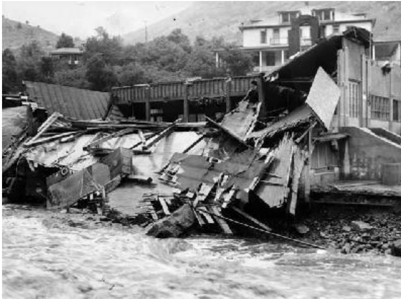
Figure 4-18 Damage to Eldorado Springs Resort, 1938 Flood
