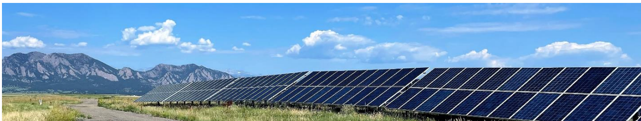
Solar Panels at the Waste Water Treatment Plant
