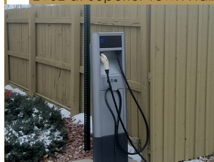
EVSE at Superior Town Hall
